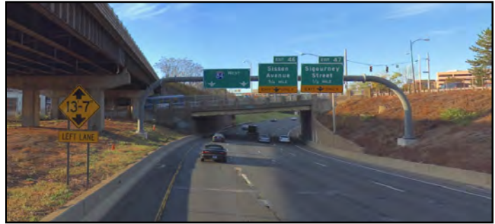
Deficient Vertical Clearance on I-84 Eastbound
